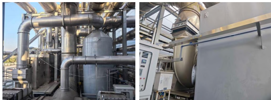
Shenzhen CSOT Semiconductor's VOCs Treatment Efficiency Enhancement Project
