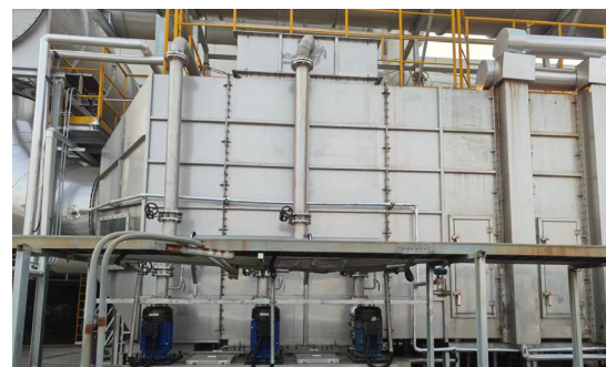
Suzhou CSOT Carries Out an Exhaust Gas Treatment Standard Upgrade Project
